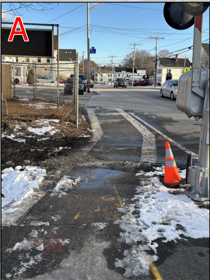
(Left) Looking east along Front St from point A, towards the municipal parking lot. The "sidewalk" is flush with the road and offers no protection for pedestrians from the traffic on Front St, which is also state route 111.
