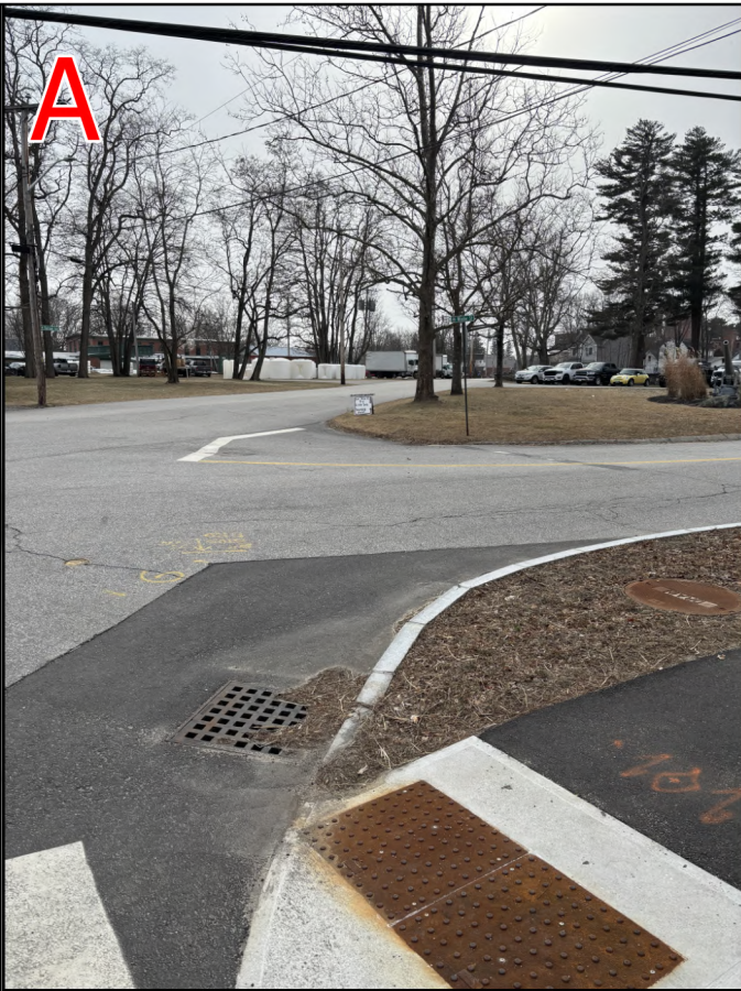
(Left) Looking south from the corner of Columbus Ave and Winter St, towards Railroad Ave. There is a crosswalk on Columbus Ave, a catch basin on the corner of Columbus and Winter St, and a catch basin on the opposite side of Winter St. This project will include a new crosswalk across Winter St, bringing pedestrians to a new sidewalk along the West side of Railroad Ave.
