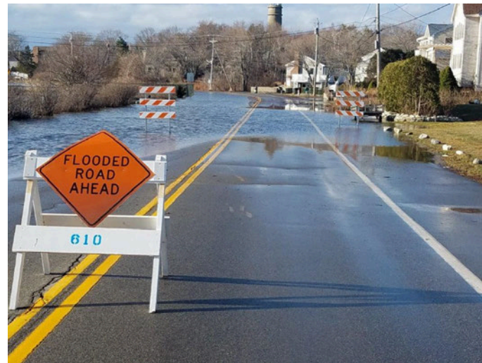
Roadway Flooding. Photo via RPC.
