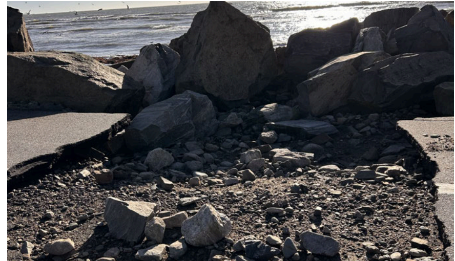
Damage to NH-1A from January 2024 flooding. Photo via NHDOT.
