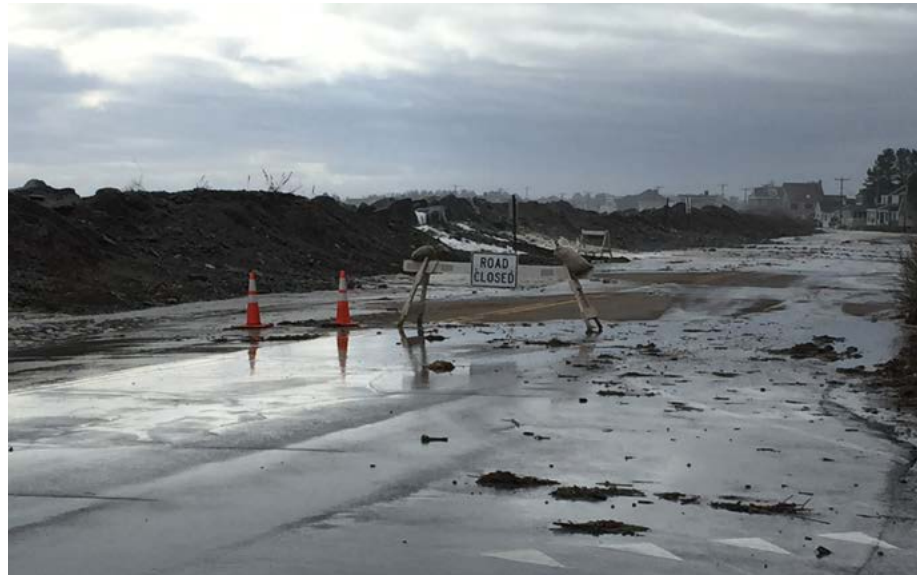
Storm Damage to NH 1A in Rye from the March 2018 Nor'easter. Photo courtesy of Tim Roache.
