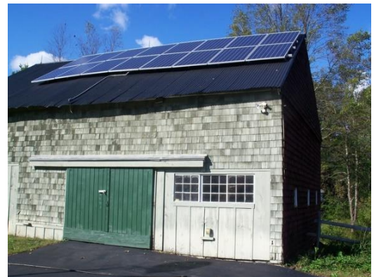
Figure EE16. Solar panel installation on an outbuilding. [Photo: SEAREI http://searei.org/seareis-photo-album/index.html ]
