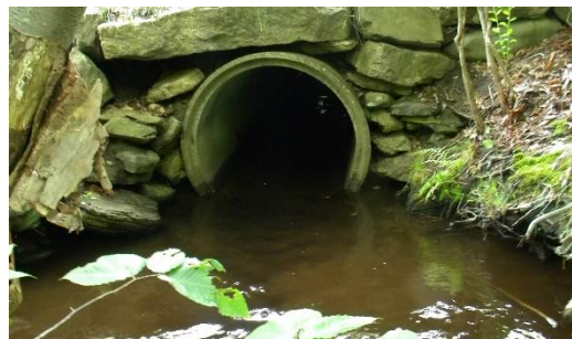
Figure NR10 - An undersized culvert in North Hampton shows evidence of being too small causing erosion on the stream bottom and banks. Photo: RPC staff.
