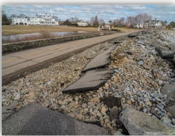
Broken walkway along the Route 1A shale piles after a coastal storm in March 2018. Photo credit: Rich Beauchesne.
