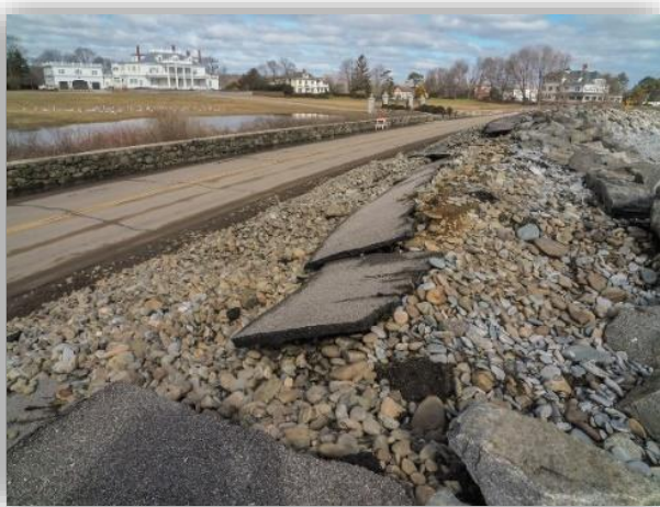
Broken walkway along the Route 1A shale piles after a coastal storm in March 2018. Photo credit: Rich Beauchesne.
