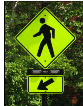
Figure 5.9: Rectangular Rapid Flashing Beacon
