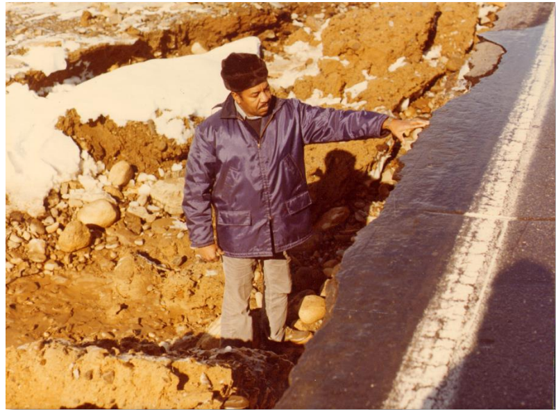
Figure 2. Selectman Aldrich Mitchell inspecting damage to Route 1A following the Blizzard of '78. [Photo Credit: Selectwoman Priscilla Jenness]
