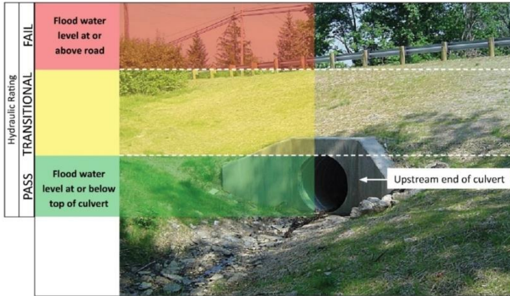
FIGURE 6: Example of how the hydraulic rating is applied to a culvert evaluation.
