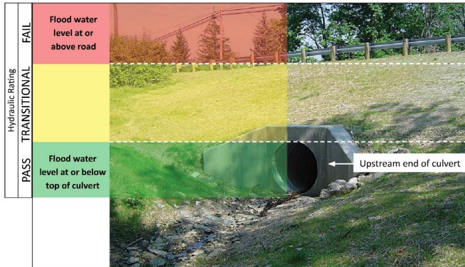
FIGURE 18: Example of how the hydraulic rating is applied to a culvert evaluation.
